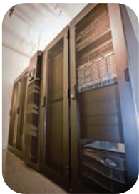
iLab Data Center
