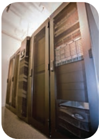
iLab Data Center
